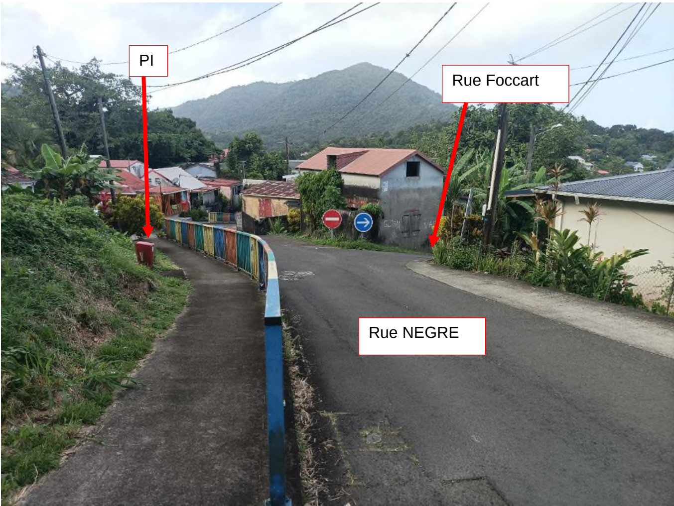
Figure 25 : Poteau incendie existant
